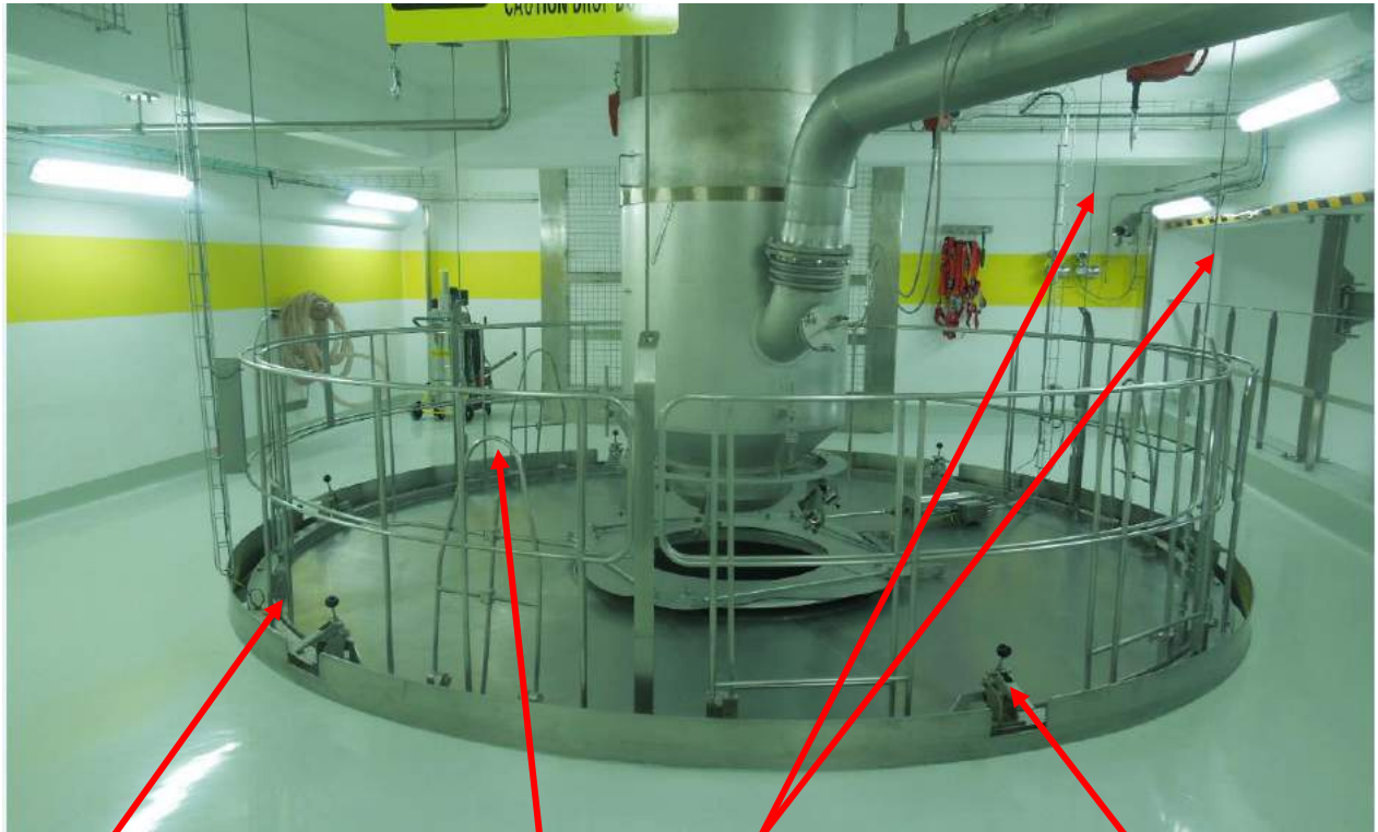
Fig. 4 Entire system with platform
