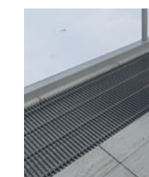
Fancoiled Heating behind a grill
