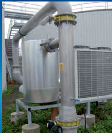
BGA Kolbermoor Station de transfert de gaz
